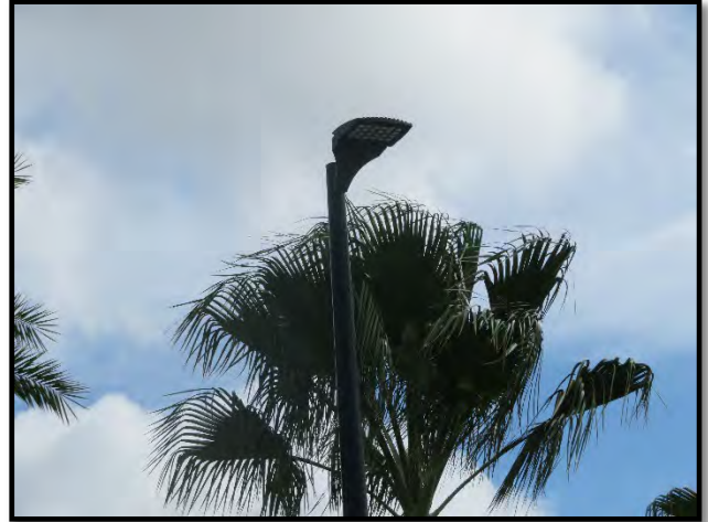
Light pole and fixture at pool
