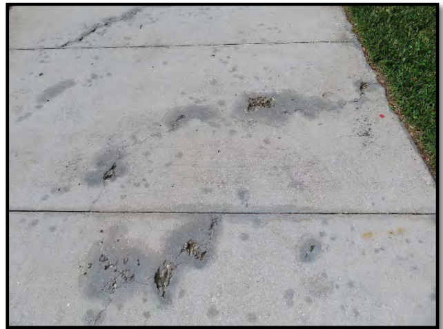
Isolated concrete spalling
