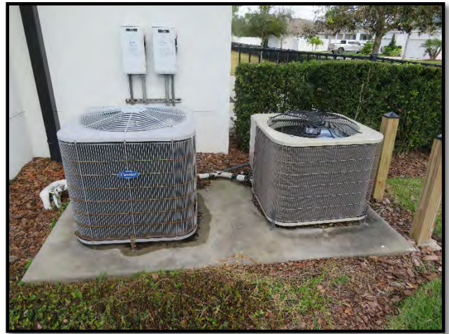
Air condensing units at Fitness Center
