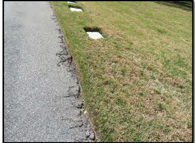
Asphalt pavement walking path edge deterioration
