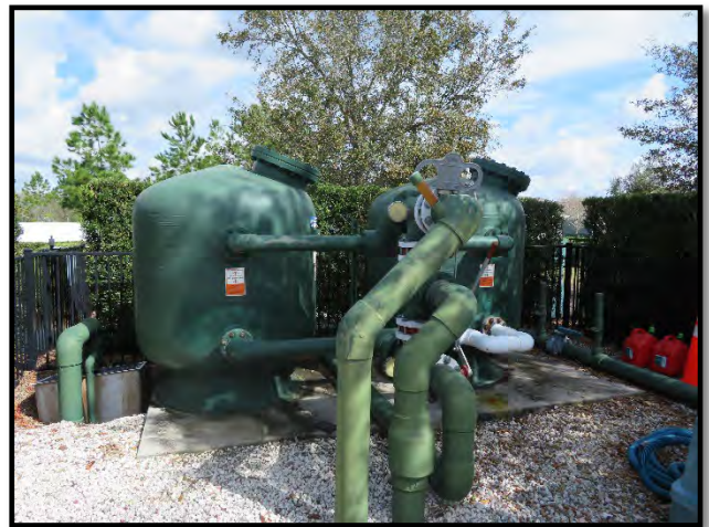
Pool mechanical equipment
