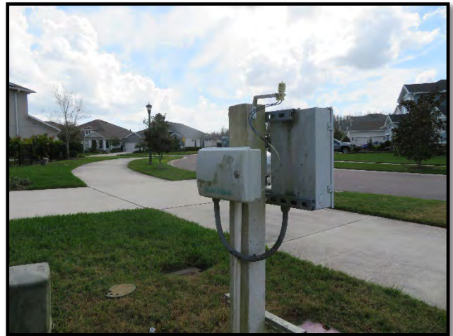
Irrigation system controller
