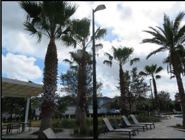
Light pole and fixture at pool
