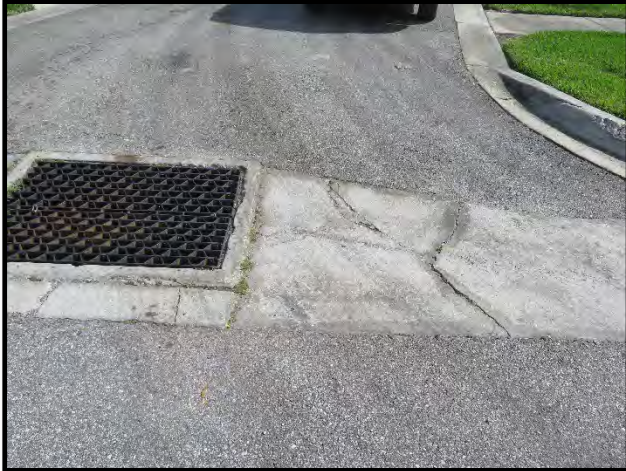
Minor settlement adjacent to catch basin
