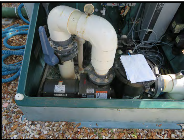
Pool mechanical equipment
