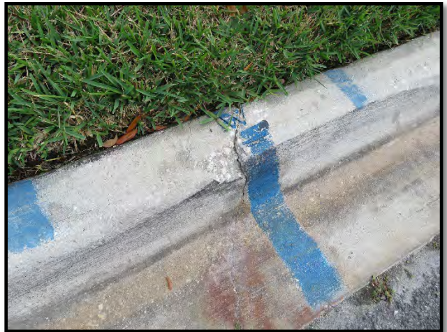
Isolated curb damage
