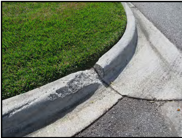
Isolated curb damage
