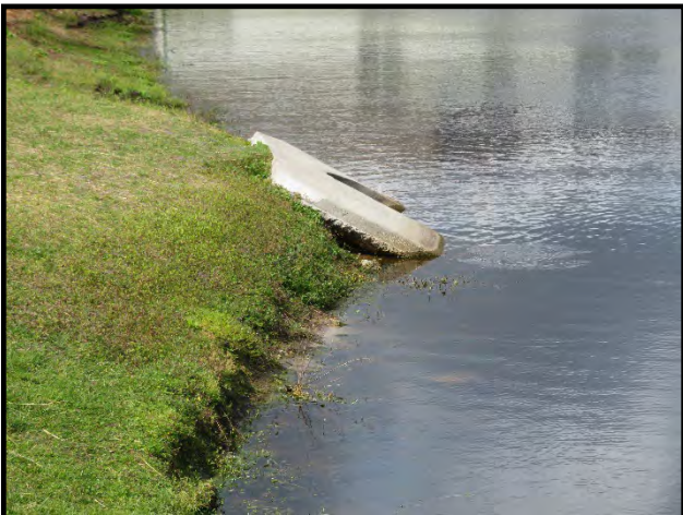
Minor settlement behind pond inlet structure
