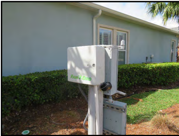
Irrigation system controller
